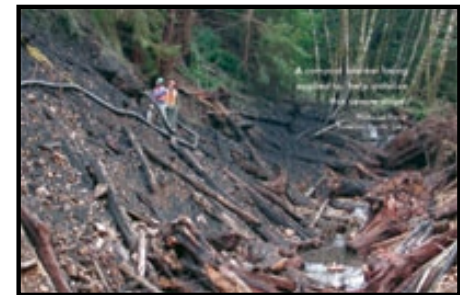
A compost blanket being applied to help stabilize this severe slope. Photo Courtesy: Peterson Pacific Corp
