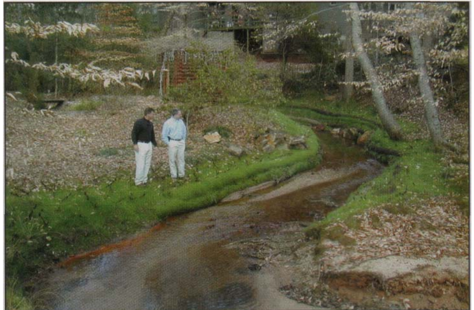
Jim Wilson & Associate review progress of the streambank stabilization project six weeks after installation.
