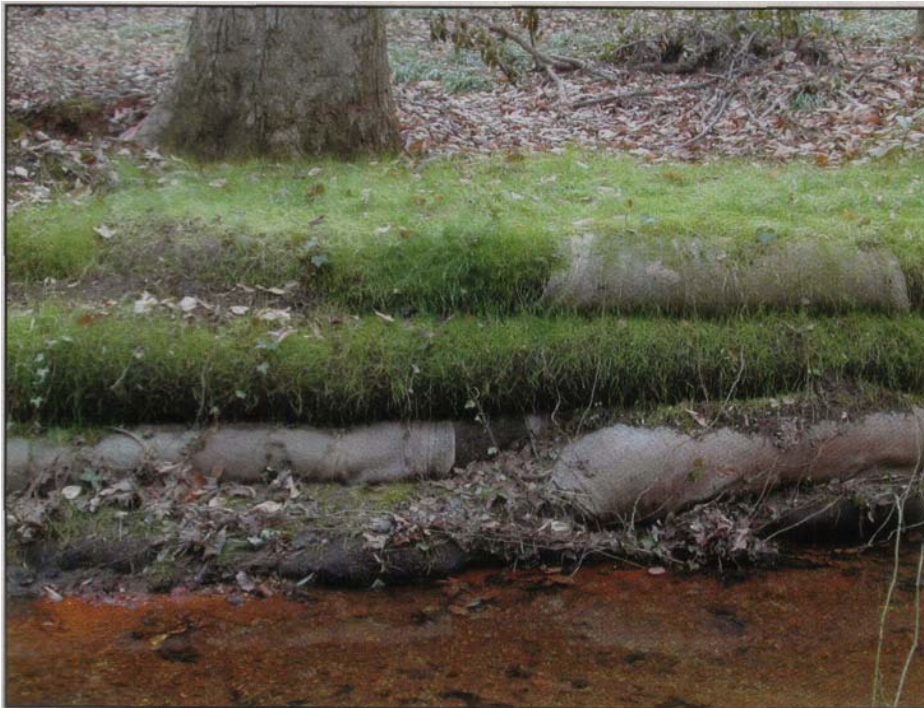
Germinating filtersocks are growing together and into the geotextile wrapped socks stacked on the banks of the creek.
