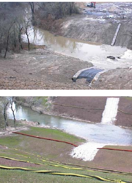
The results of applying compost to stabilize a stream bank slope is evident in these "before and after" views.
