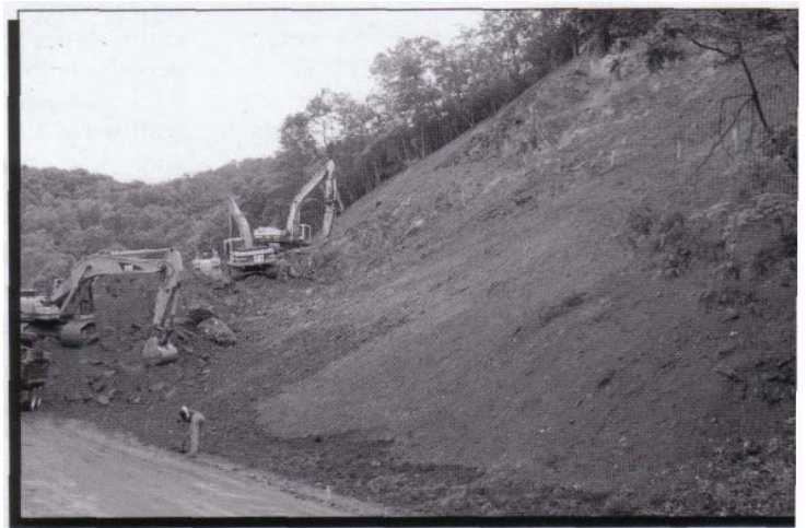
The excavation of the slope prior to the placement of compost had proceeded well by June 4, as shown in this photo of clearing the slide material.
