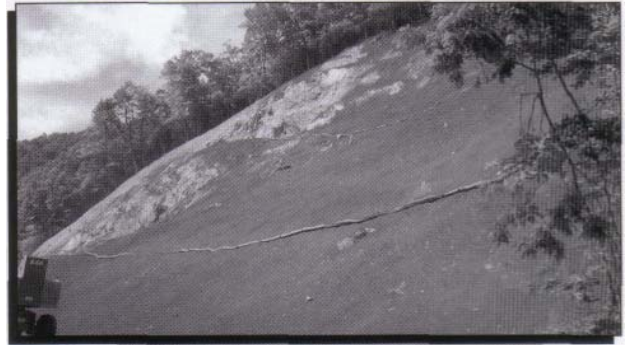
By June 26, the contractor had begun spreading the compost with the seed mixture on the completed slope. The berm, constructed of a sock containing compost, controls water runoff.
