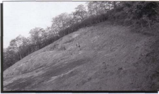
By June 17, the contractor's rock climbers were rappelling down the slope to place lockdown netting to help hold the compost in place until a mature root mat is established.
