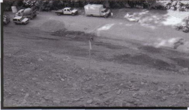
Looking down the slope across the lockdown netting to the Blue Ridge Parkway below.
