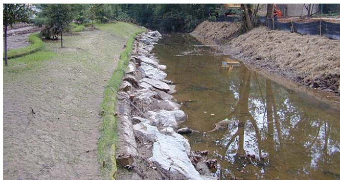
A stream bank restoration project in the city of Atlanta incorporated compost blankets and contained berms (left half of photo). The picture shown is after a flood totally submerged the restored area in water.
